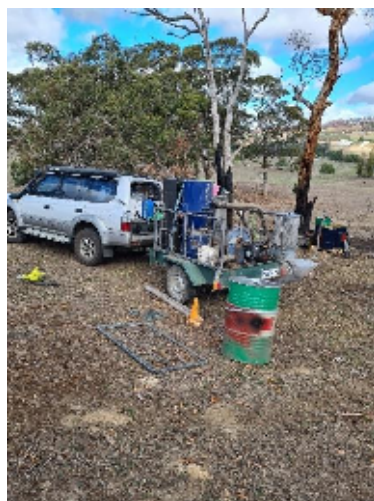
Ash Pump and Containers
